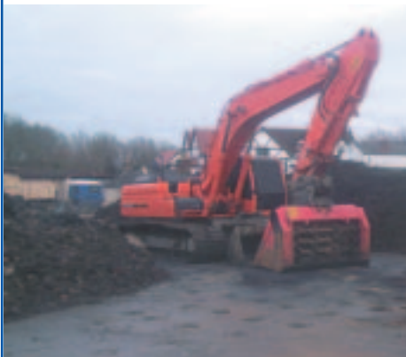
Ex-situ mixing of cadmium contaminated soils was part of the sustainable remediation solution
